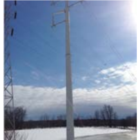
Fig. 5: A weathering steel transmission pole.
