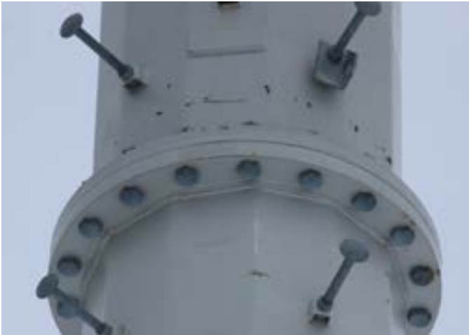
Fig. 6: Photograph showing mechanical damage to paint.
