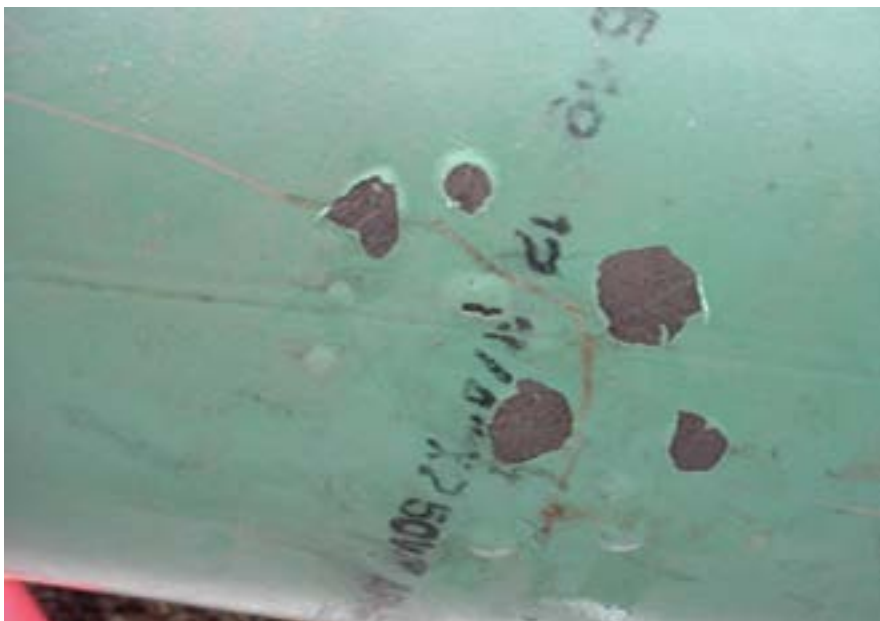
Fig. 1: Blistering of FBE coating on steel pipe. Figures courtesy of the authors unless otherwise noted.
